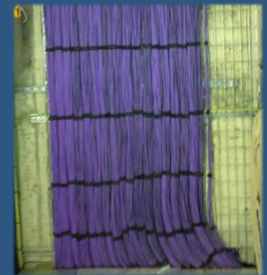
Over 40 kilometres of Cat 6 cable were purchased for installation on the project
